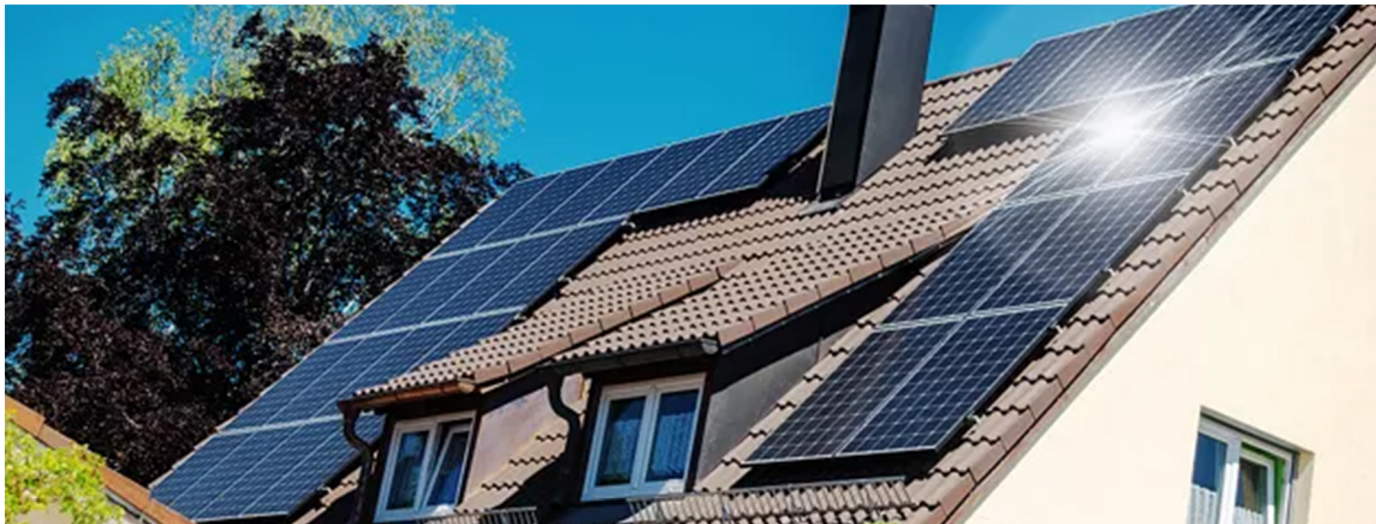
550 kW Rooftop PV Plant In Berlin, Germany
